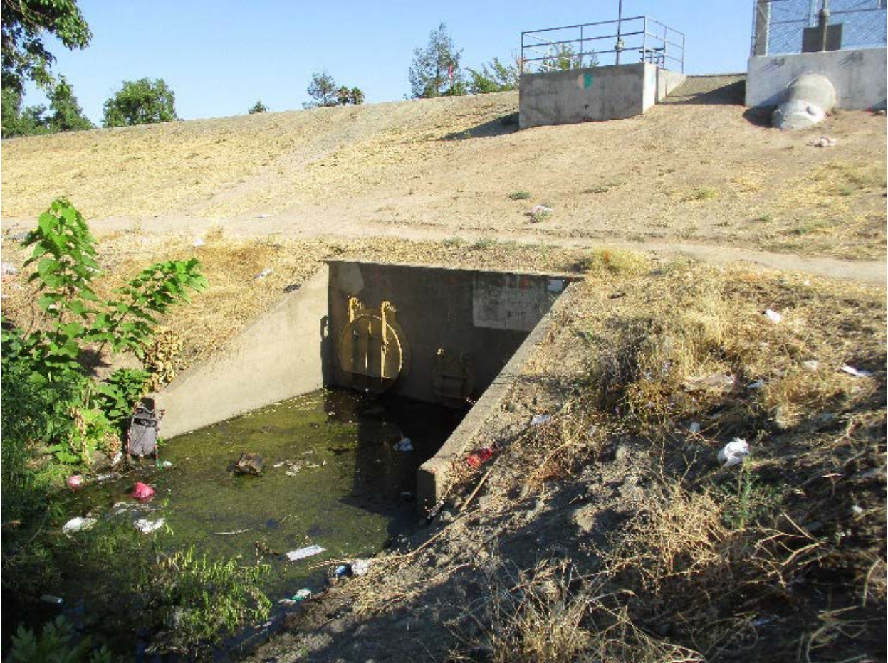
Figure 3: View looking northwest toward the Sump 103 outfall as it enters Arcade Creek
