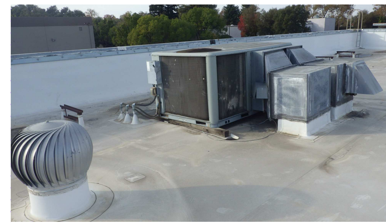
UNIT B DEMO EXISTING HVAC UNIT, PIPE & CONDUITS, AND DUCT WORK. PATCH HOLES IN (E) ROOF & PREP FOR INSTALLATION OF NEW UNIT WITH NEW PIPE, CONDUIT & DUCT PENETRATIONS.
