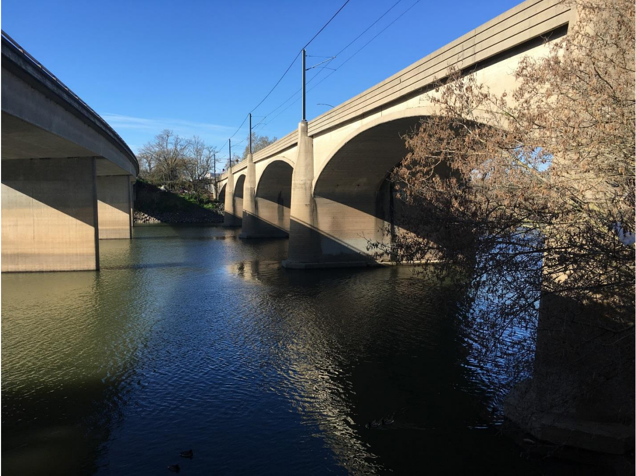
Figure 4. 1 - View of the 12 th Street Bridge (right) and the 16 th Street Bridge (left) along State Route 160 across the American River. This view is looking south-west. In this view Abutment 1 (south bank) can be seen, as well as Piers 2, 3, 4, and 5. Abutment 6 (north bank) is not shown. A federal levee exists along the south bank but not along the north bank.
