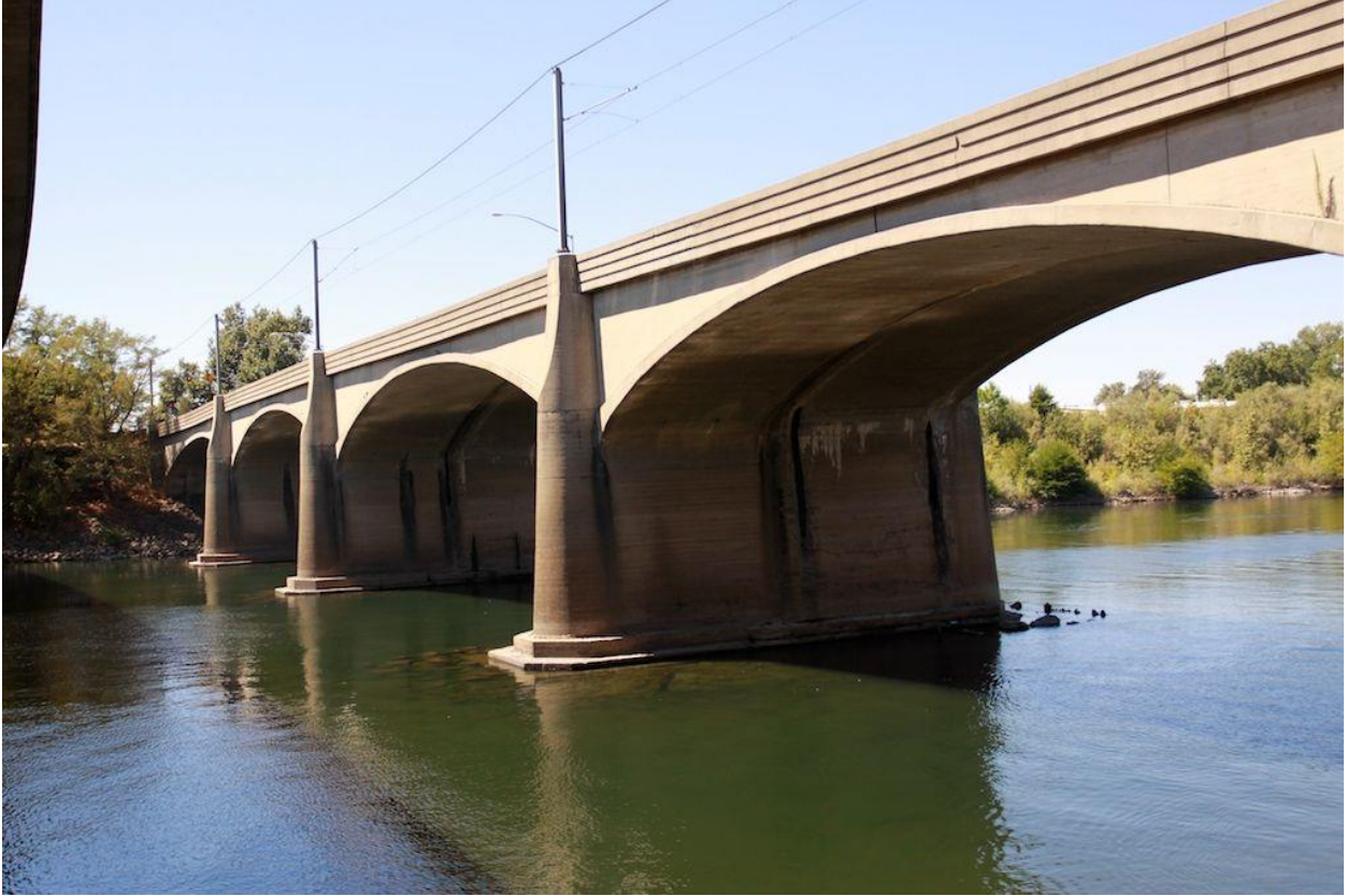
Figure 4. 2 – View of the 12 th Street Bridge on state route 160 across the American River from the east side. This view is looking south-west. The south bank, where the federal levee is located, has existing rock slope protection.
