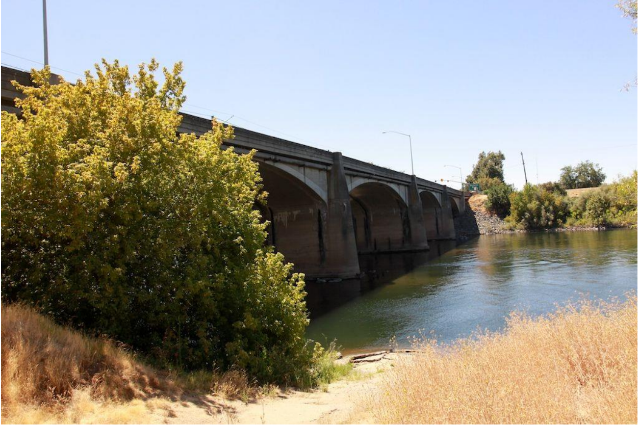
Figure 4. 3 - View of the 12 th Street Bridge on state route 160 across the American River from the west side. This view is looking south. The south bank, where the federal levee is located, has existing rock slope protection. Also seen is the existing north bank which does not feature a levee.
