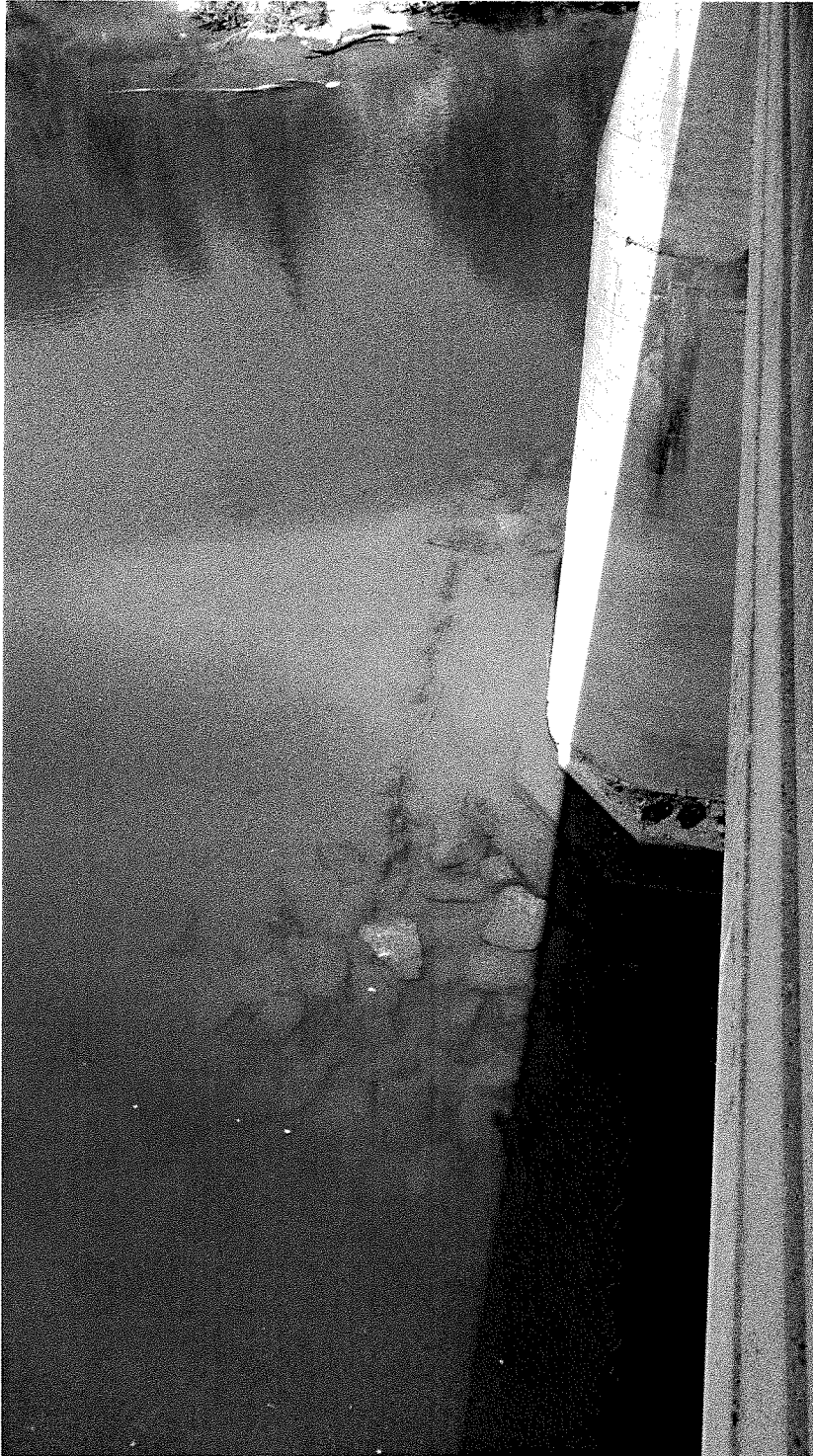
Figure 4. 4 – Example of the existing rock slope protection that will be removed and replaced with new permanent sheet piles. Some of the existing rock slope protection has been carried away while some remains in place. This photo is showing the downstream portion of the pier.
