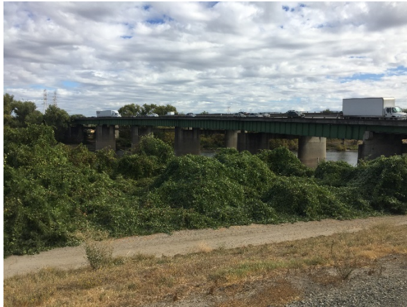
1: GROUND LEVEL PHOTO LOOKING AT AMERICAN RIVER BRIDGE FROM THE RIVER LEVEL.
