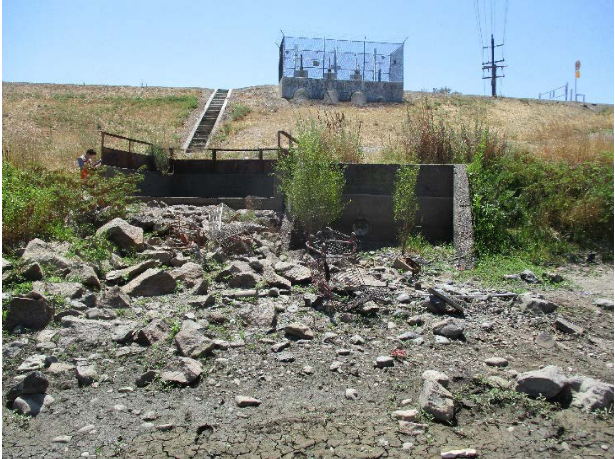
Figure 3: View looking south toward the Sump 154 concrete outfall structures from the dry bed of Arcade Creek.
