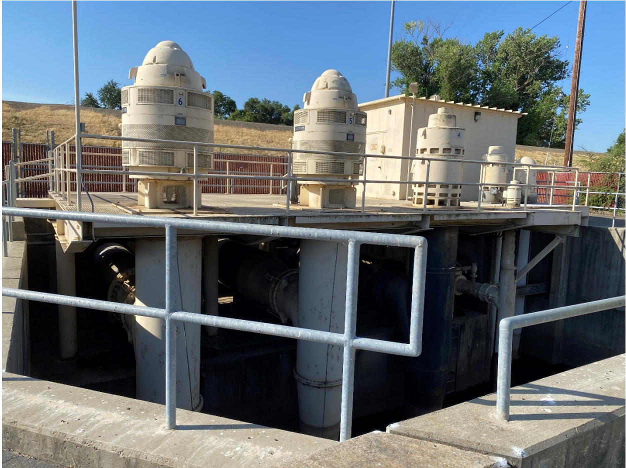
Figure 1: View of pump station
