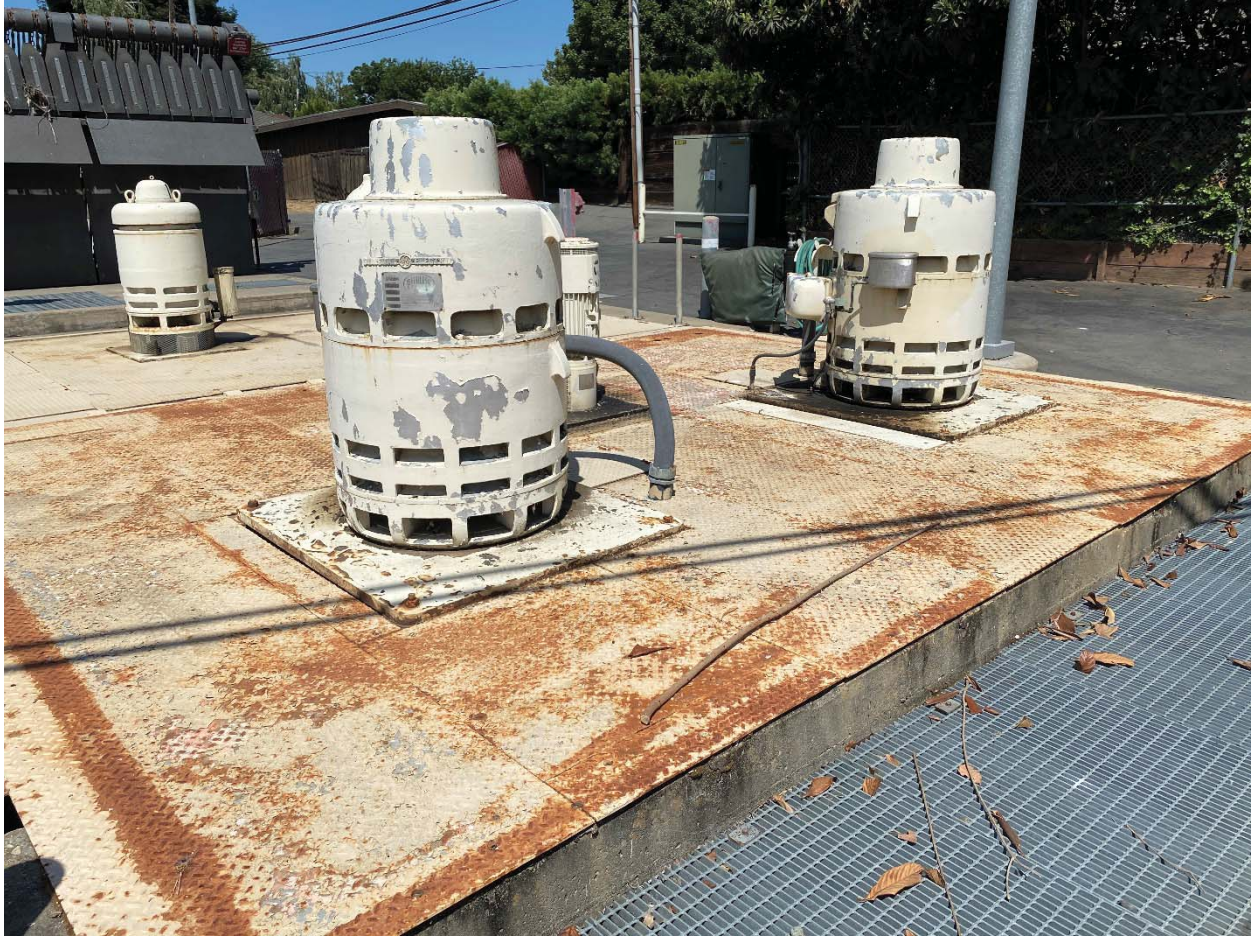
Figure 1: View of pump station
